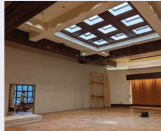
The Allen Whitehill Clowes Sculpture Court, showing the temporary wall during construction.
